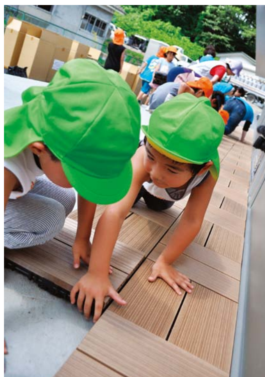
Children helping to make a deck in the temporary childcare center ©JCU
