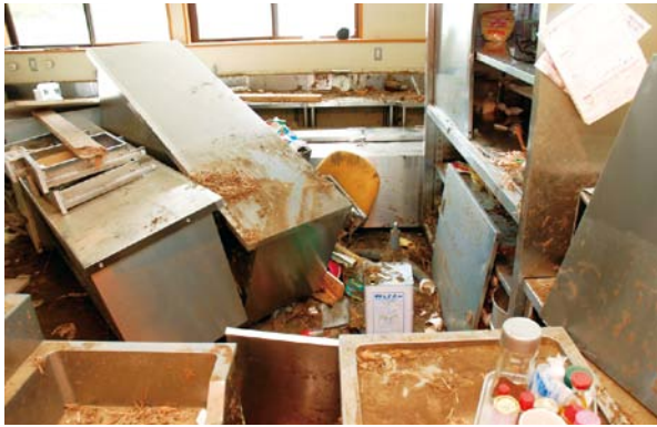
The tsunami-affected kitchen in a nursery school Photo provided by a nursery school in Rikuzentakata city
